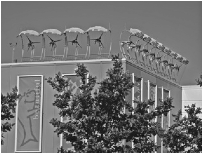
FIGURE 9.6 Twelve 1-kW wind turbines mounted on parapet of building. (Photo courtesy of AeroVironment.)
